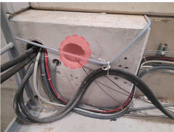
Figure 3: Pos 2 : The cable path exit of the labyrinth.
